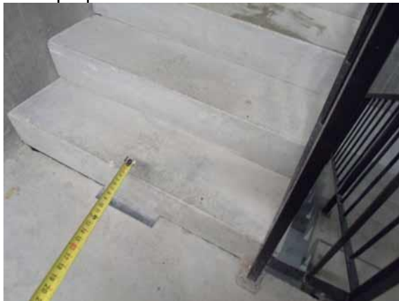
Properly mark the edge of the steps
