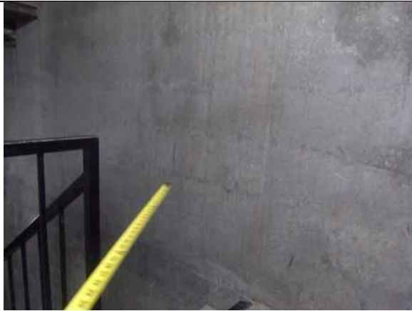
Provide proper handrails and handrail extensions
