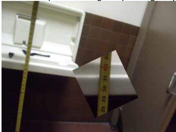
This changing table height is compliant
