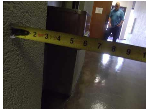
Provide proper barrier for the drinking fountains typical of all
