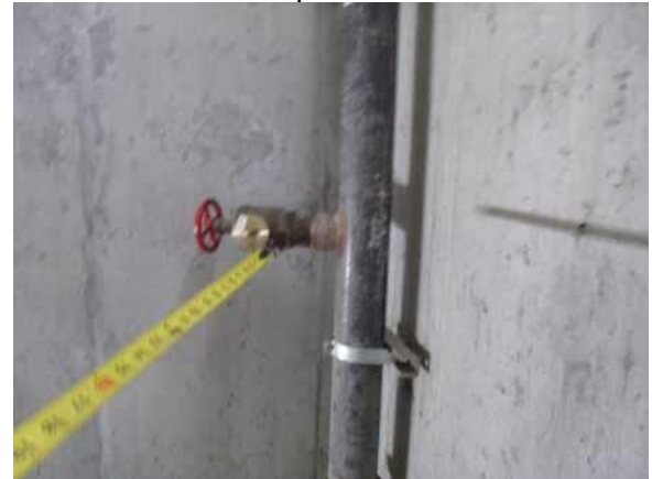
Provide cane detection under protruding connection
