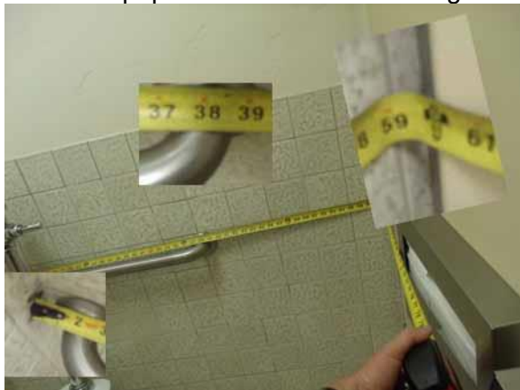
Stall width and rear grab bar are not compliant
