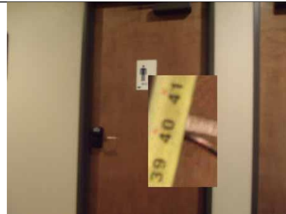
This door handle height is compliant
