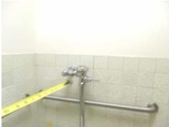
This plumbing obstructs the rear grab bar
