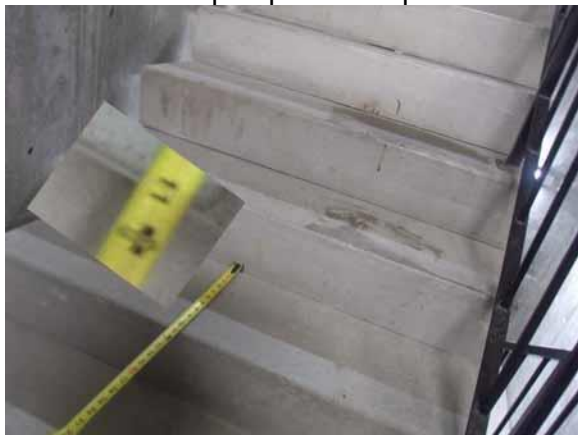
The step depth is compliant
