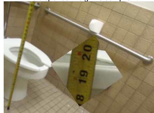
This toilet seat height exceeds 19" maximum
