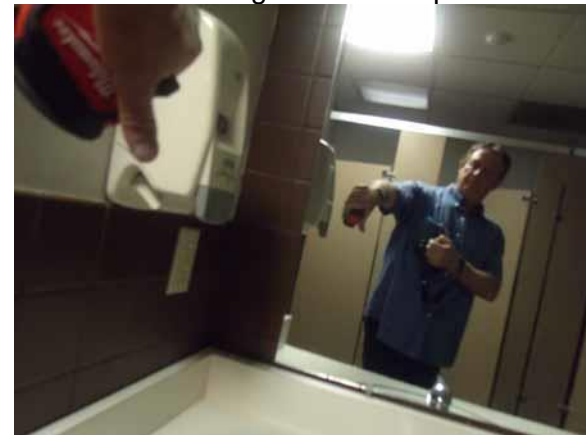
This paper towel dispenser exceeds 40" high
