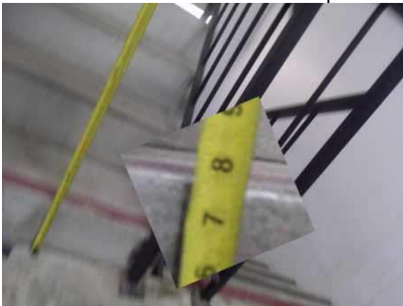
This riser height exceeds 7" high
