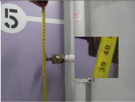
Fire hose connection protrudes into the circulation path
