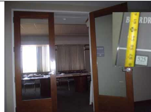
Maintain proper braille room identification signs
