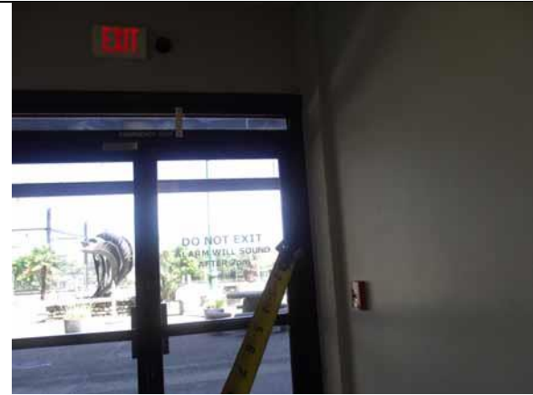
Provide proper exit braille signage Typical of all exit doors
