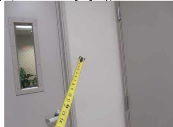
Provide proper signage for the stairs Typical of all stair doors
