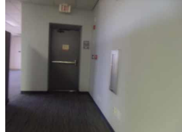
This exit stair sign is not compliant
