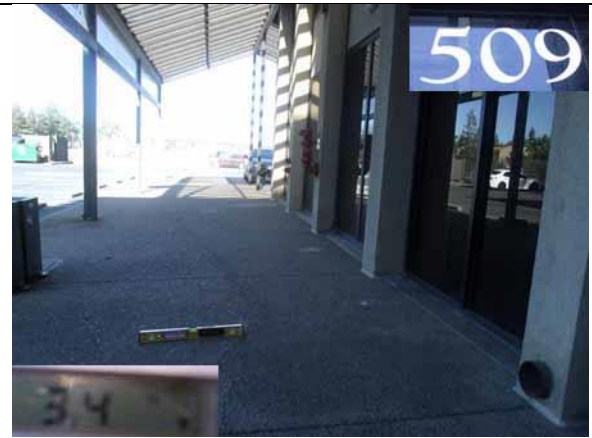
This section of cross slope exceeds 2.08%
