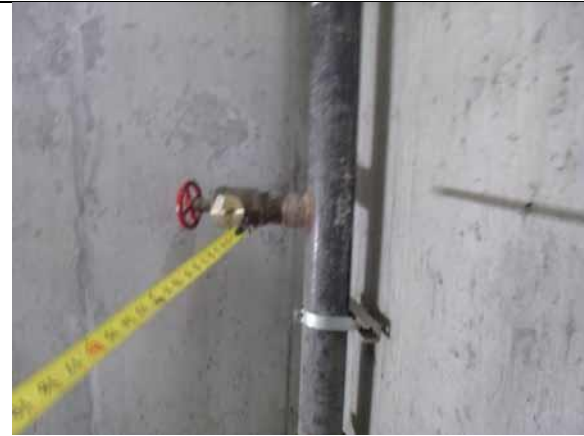
Provide cane detection under protruding connection
