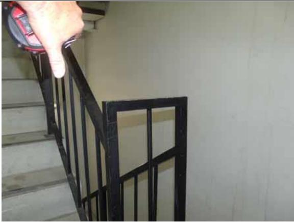
Handrail extensions are not compliant
