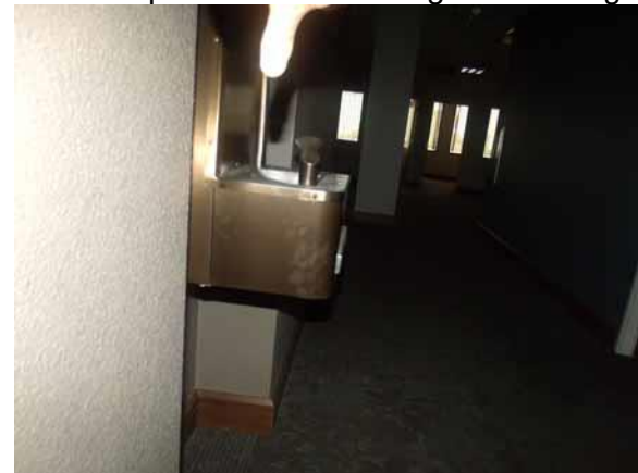
There is no barrier for the drinking fountain
