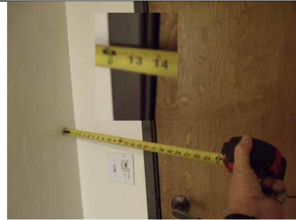
This pull side is not 18" wide minimum
