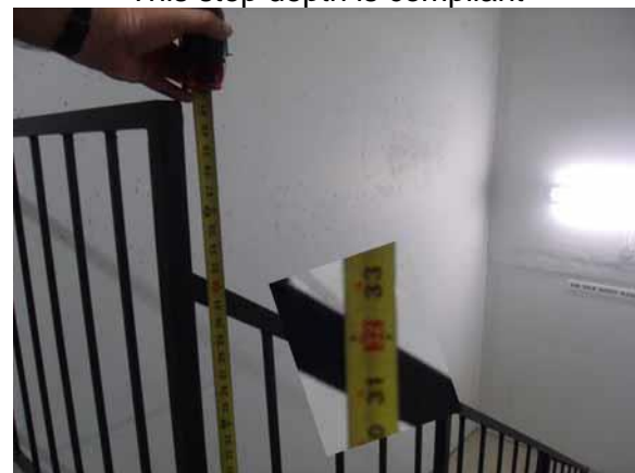
This handrail height is compliant/size is not compliant
