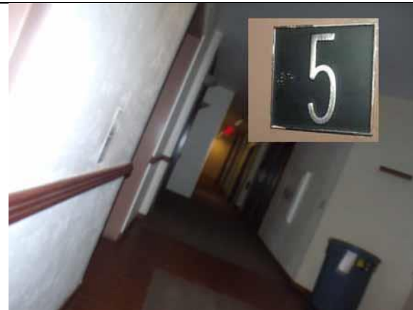
Elevator floor number exceed 60" high
