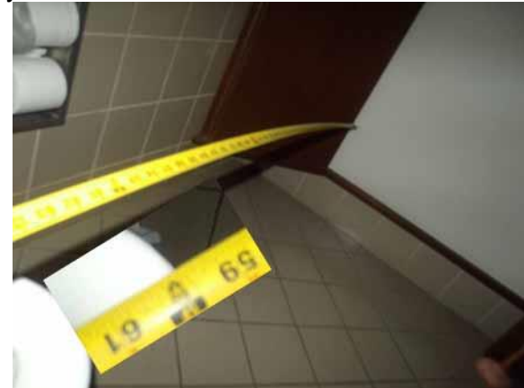
This clear area is compliant without the storage cabinet
