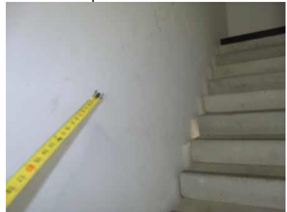
Handrails are not provided on both sides of the stairs
