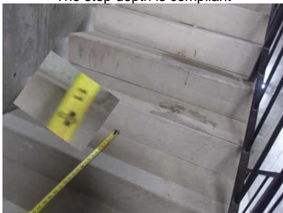
The step depth is compliant
