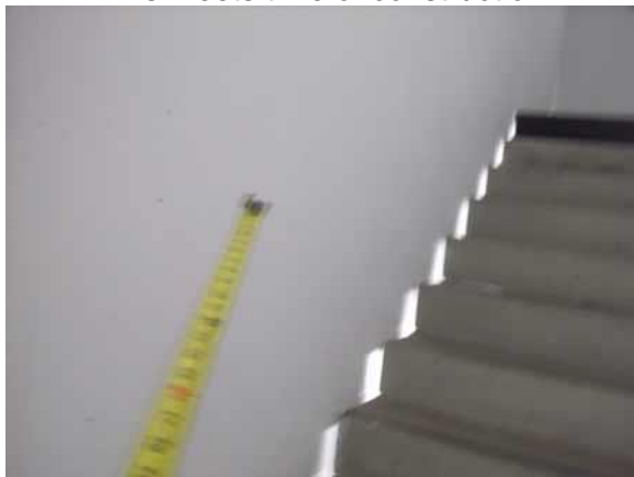
Provide handrails on both sides of stairs
