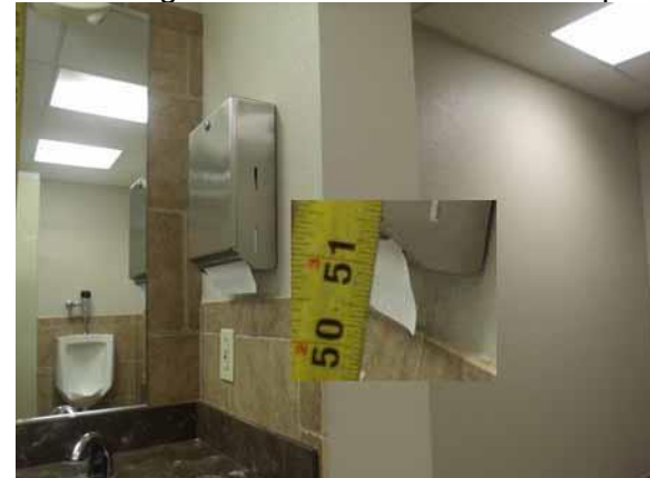
This dispenser exceeds 40" high to operable parts
