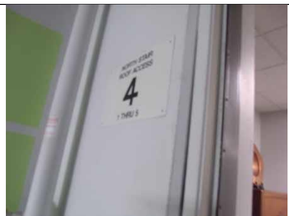
Provide proper floor identification sign
