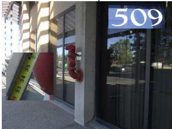
Provide cane detection under the fire riser connection
