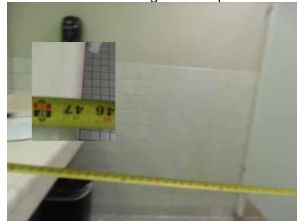
This requires 48" on pull side of door
