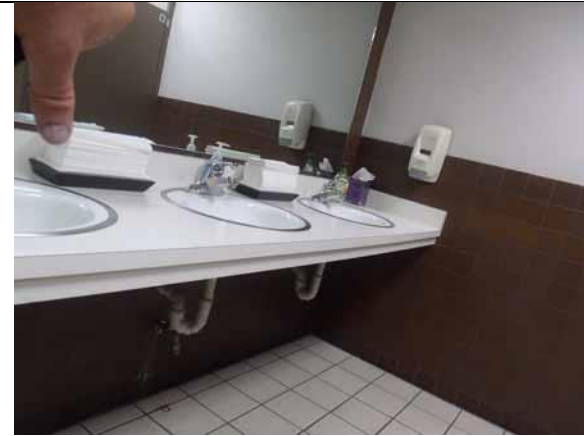
This lav counter height does not provide proper knee clearance
