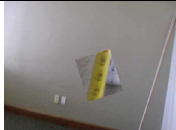
This outlet height is compliant
