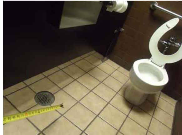
Repaor the floor slope that exceeds 2.08% maximum allowed
