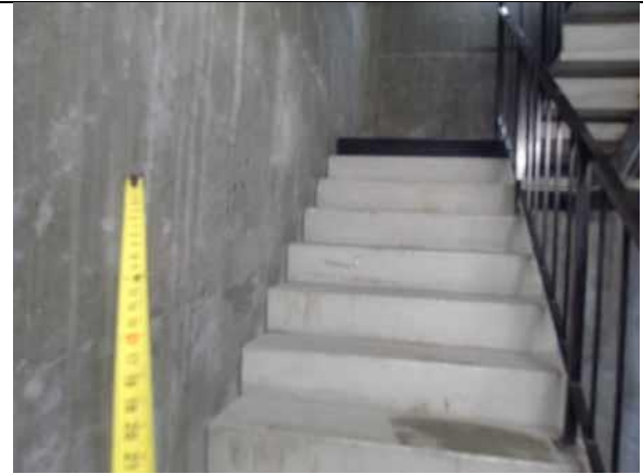
Handrails are not provided on both sides
