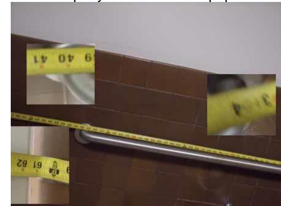
Properly locate the rear grab bar/stall width is compliant
