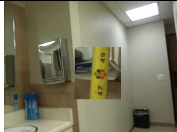
This dispenser exceeds 40" high to operable parts
