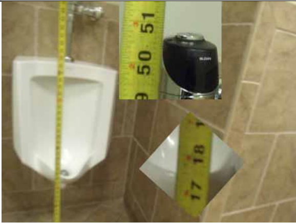
This urinal height exceeds 17" to top of the rim
