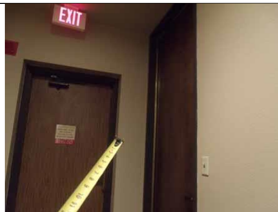
Provide proper stair exit signage
