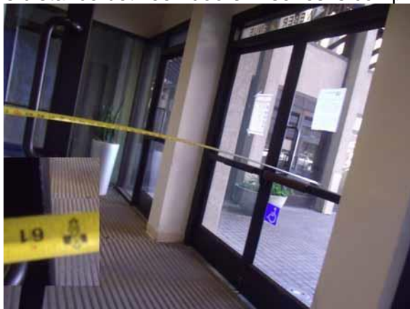
This distance between doors in series is compliant
