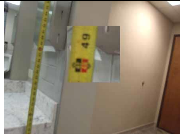
This dispenser height exceeds 40" high to operable parts
