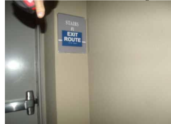
Provide proper exit stair signs
