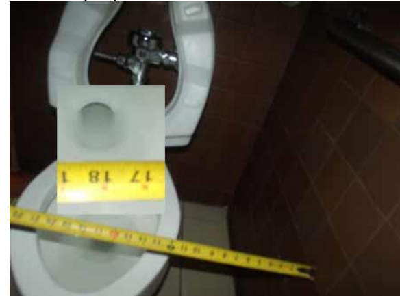
This toilet offset is compliant
