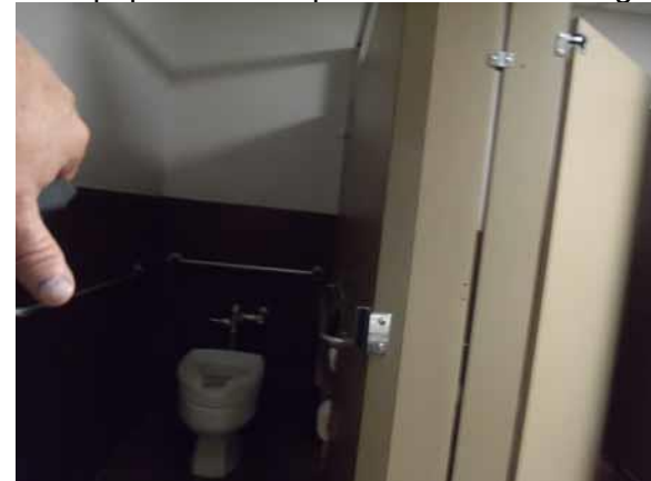
This stall is not compliant/remove stall panels and make single user
