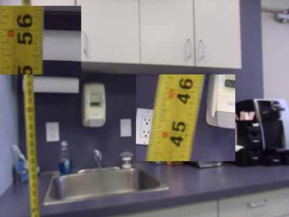
Dispenser at the counters shall meet reach range requirements
