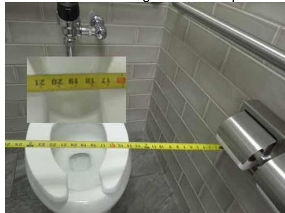
This toilet offset exceeds 18" to center from wall
