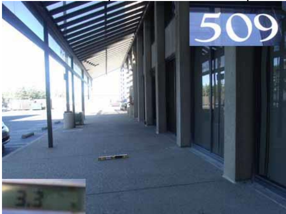
This section of cross slope exceeds 2.08%
