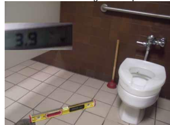
Repair the floor slope to be 2.08% maximum
