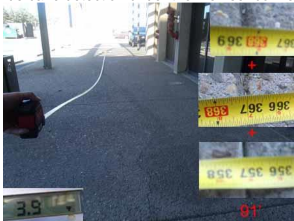
This is the length of route that needs repaired
