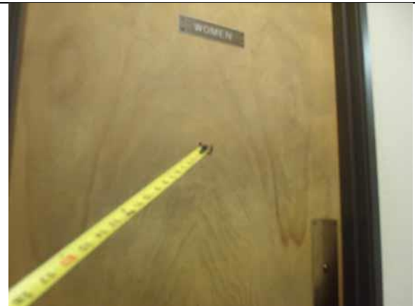
Provide proper door signage
