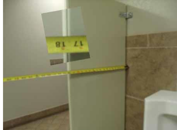
This panel length is compliant
