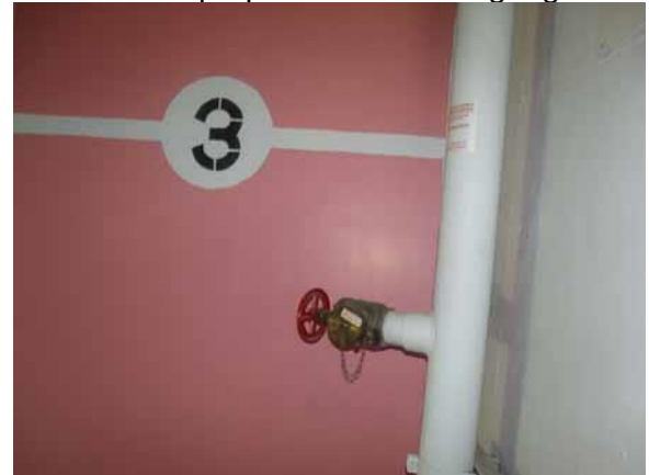
Provide cane detection at the sprinkler riser hose connection
