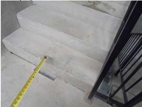
Properly mark the edge of the steps
