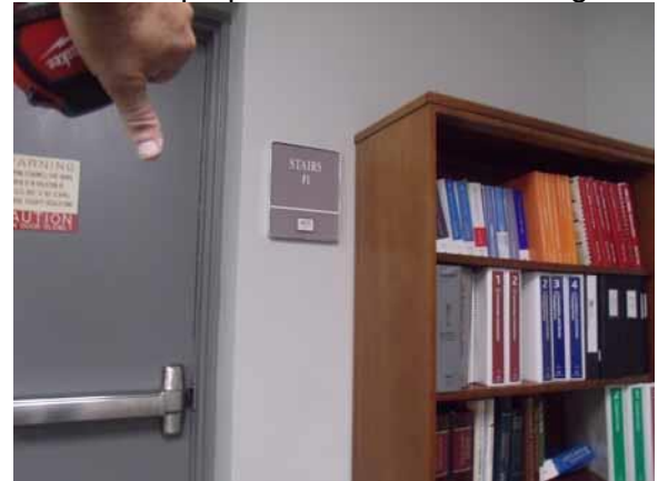
Provide proper stair exit signage
