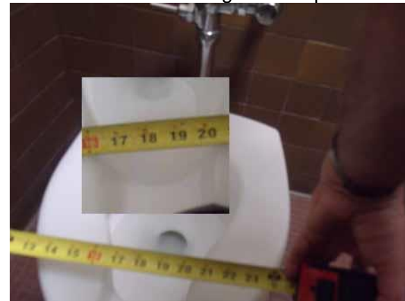
This toilet offset is compliant
