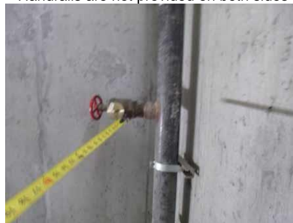
Provide cane detection under protruding connection
