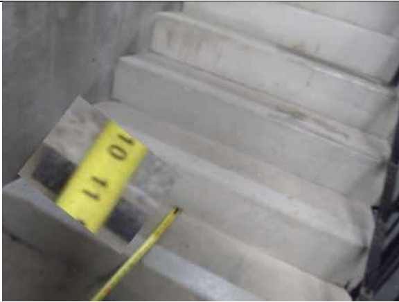
The step depth is compliant
