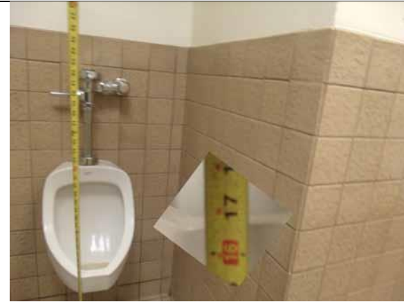
This urinal height is compliant
