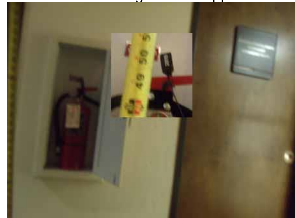
This fire extinguisher height is compliant
