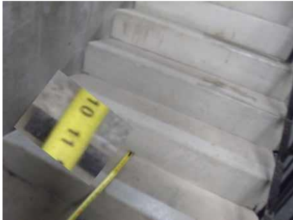
The step depth is compliant
