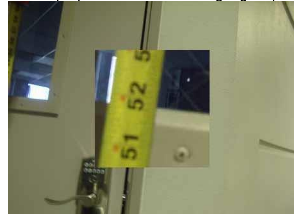
Viewing windows exceed 43" above the floor typical
