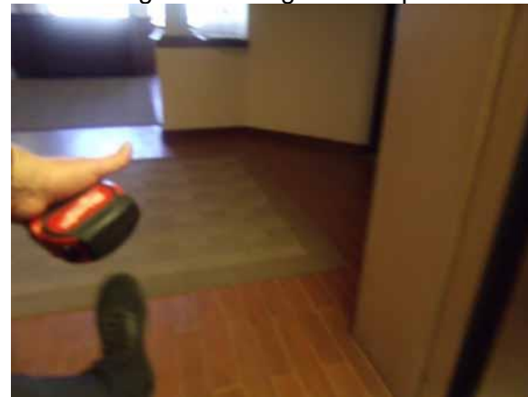
The automatic door opener works
