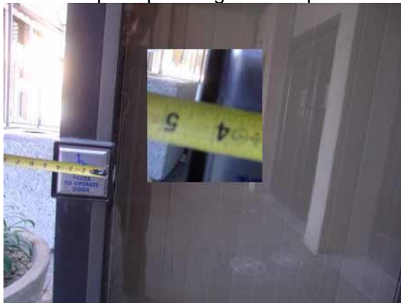
This push pad is compliant
