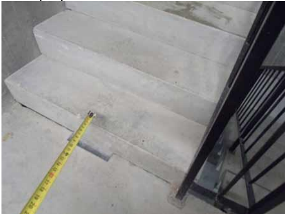
Properly mark the edge of the steps
