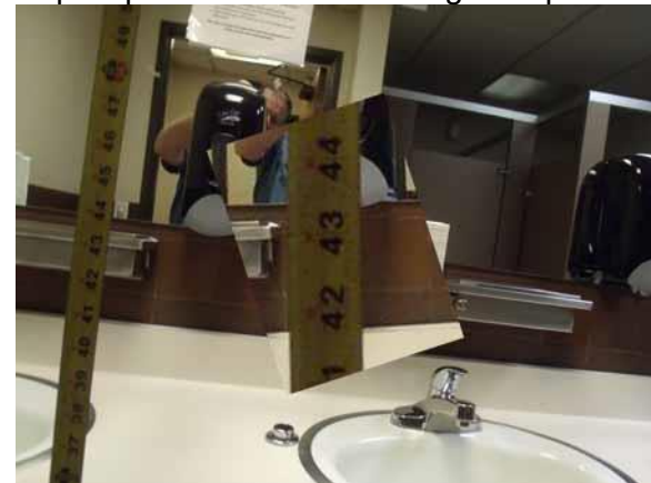
This mirror height exceeds 40" high to reflective parts
