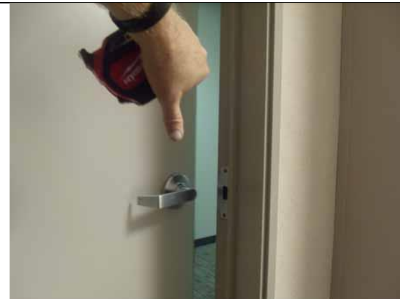
This door closing speed exceeds allowable
