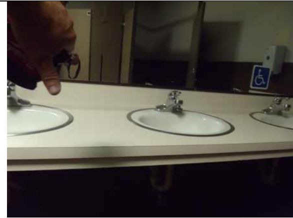
This lav height is not compliant
