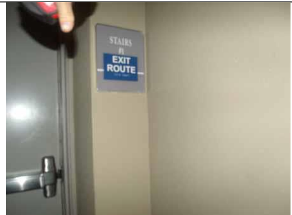
This stair exit sign is not compliant
