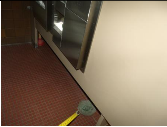
Repair the floor slope that exceeds 2.08%
