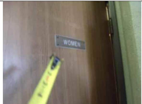
Provide proper door sign
