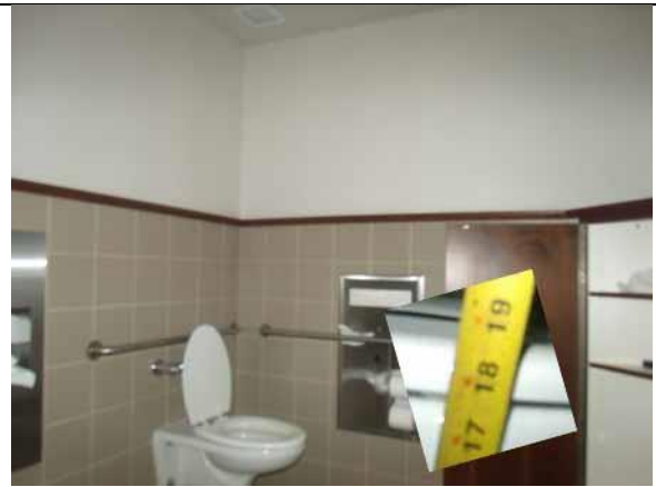
This toilet height is compliant
