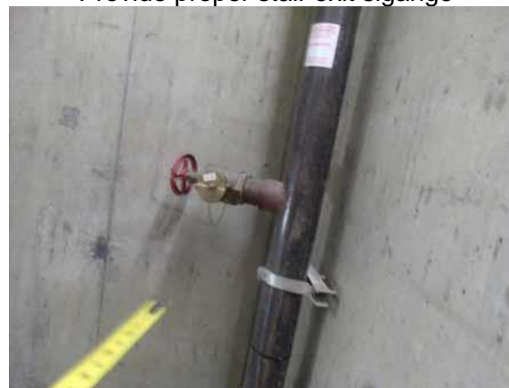
Provide cane detection for protruding valve
