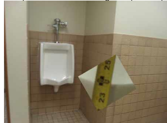
This urinal height exceeds 17" to top of rim
