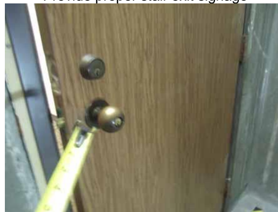
Provide proper door handle
