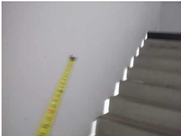
Provide handrails on both sides of stairs
