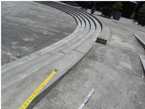
This ramp does not have handrails
