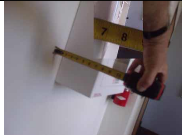
Provide cane detection under AED due to protruding more than 4"
