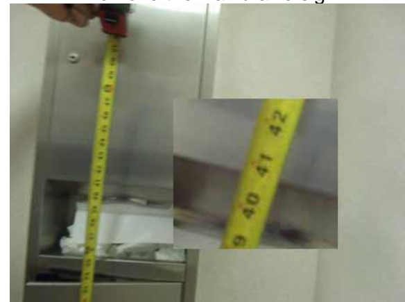
This paper towel dispenser exceeds 40" high
