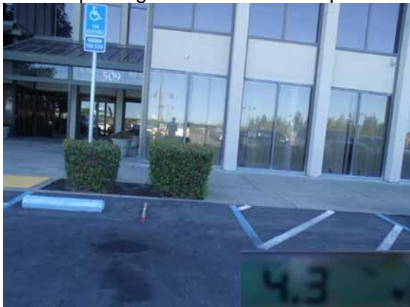
This section of slope exceeds 2.08% maximum allowed
