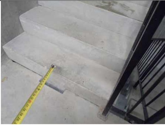
Properly mark the edge of the steps
