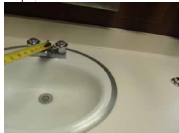
These faucet handles require pinching and twisting to operate
