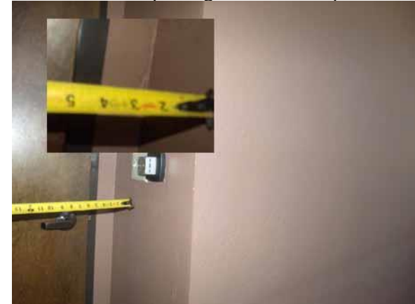
Relocate door for N/W office for proper side clearance
