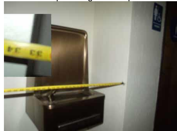
Provide full depth barrier for the drinking fountain
