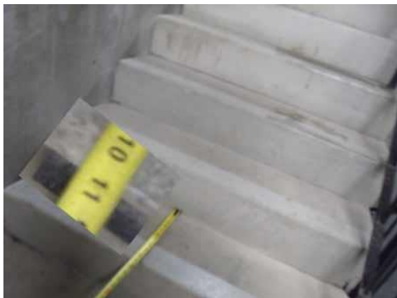
The step depth is compliant
