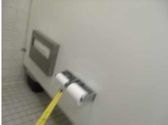
Properly locate the toilet paper
