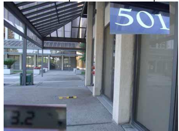
This section of cross slope exceeds 2.08%
