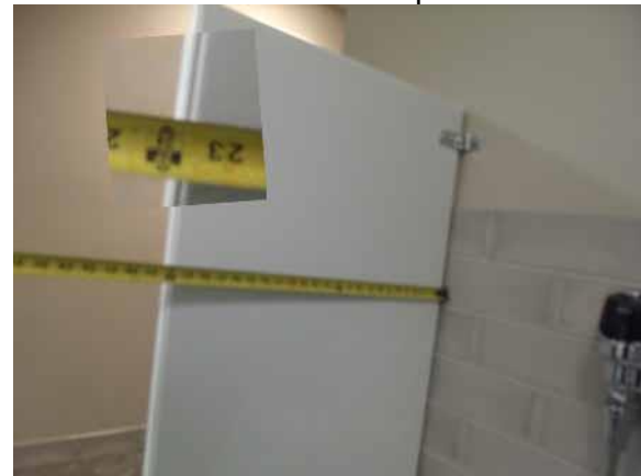
This depth is compliant
