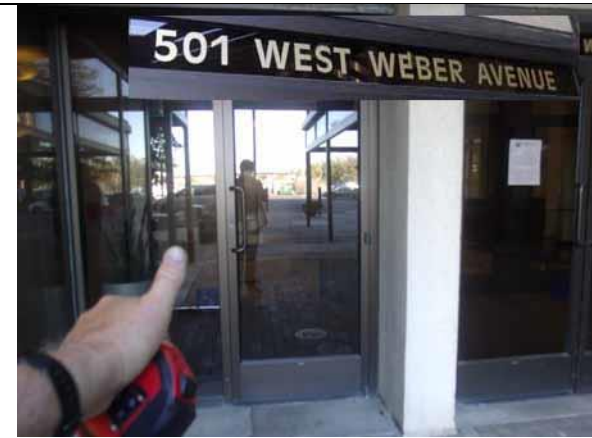
This power assisted door is functional
