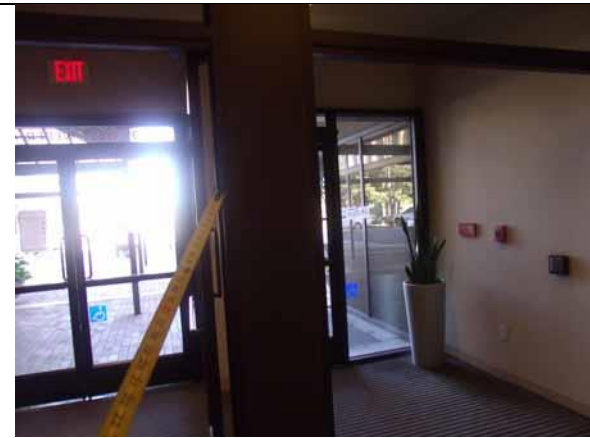
Provide proper exit braille signage Typical of all exit route doors
