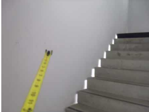
Provide proper handrails on both sides of stairs
