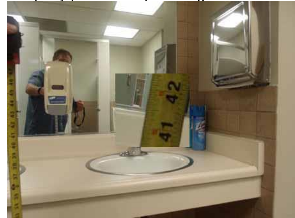
This soap dispenser exceeds 40" high to operable parts
