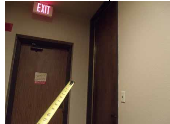
Provide proper stair exit signage
