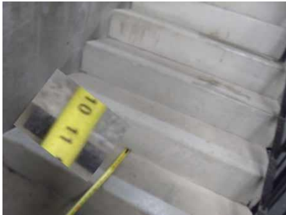
The step depth is compliant
