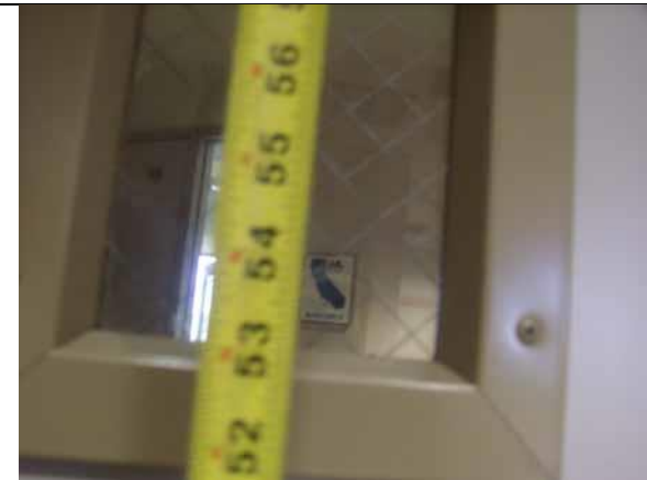
Viewing windows exceed 43" above the floor typical
