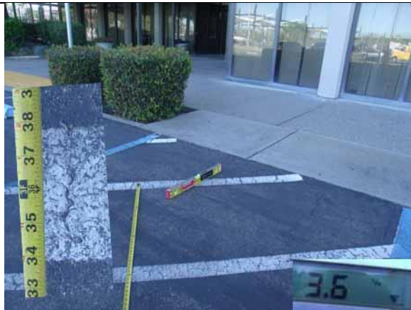
This section of slope exceeds 2.08% maximum allowed
