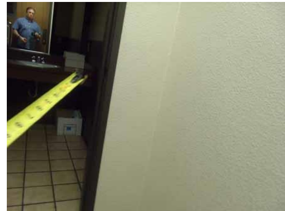
Not adequate clear areas for inner door
