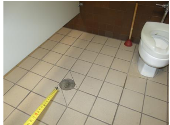
Repair the floor area where it exceeds 2.08% maximum slope
