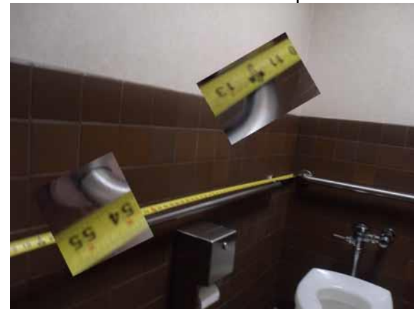
This side grab bar placement is compliant
