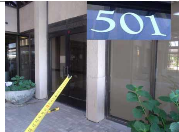
Provide signage directing to the accessible entrance door
