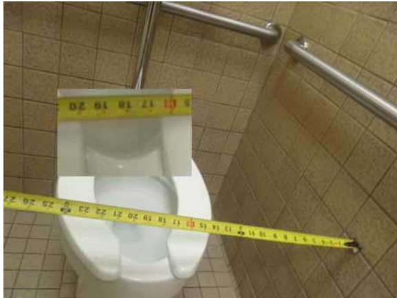
This toilet offset is compliant
