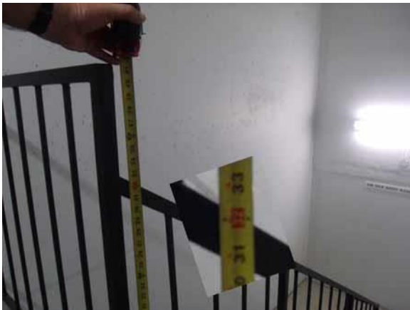
Handrail size is not compliant
