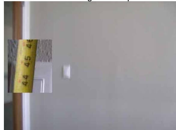
This switch height is compliant
