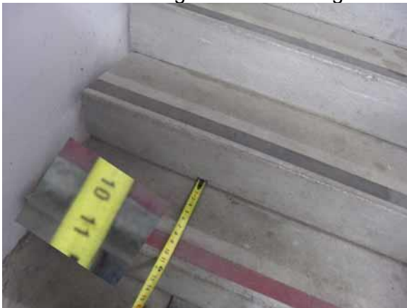
The step depth is compliant
