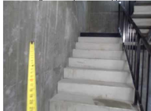
Handrails are not provided on both sides
