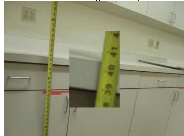
This counter exceeds 36" high
