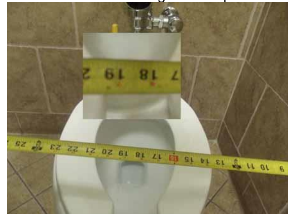
This toilet offset is compliant
