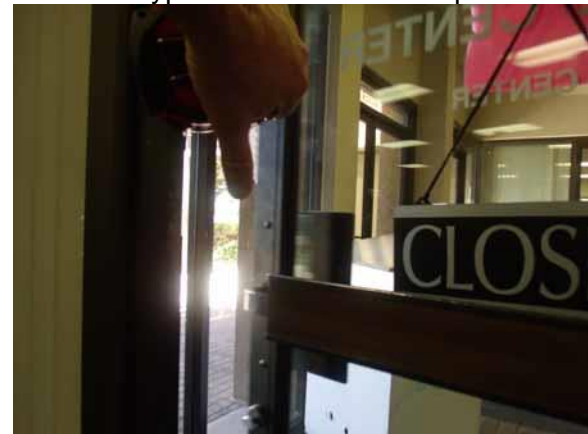
This door operation forces exceeds allowable
