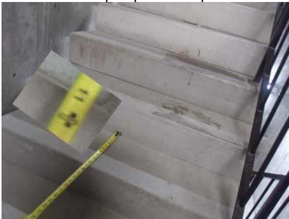
The step depth is compliant
