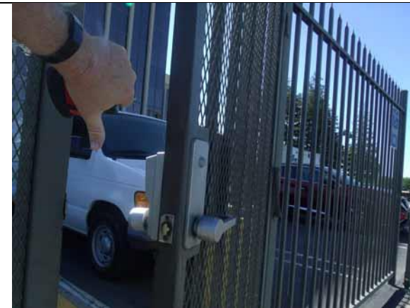
This door closing speed exceeds allowable
