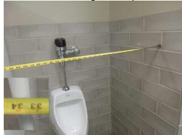
This width is compliant
