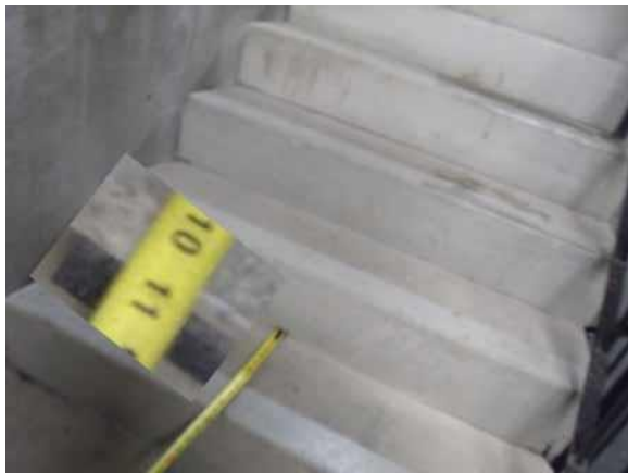
The step depth is compliant
