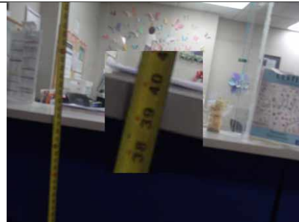
This counter height exceeds allowable
