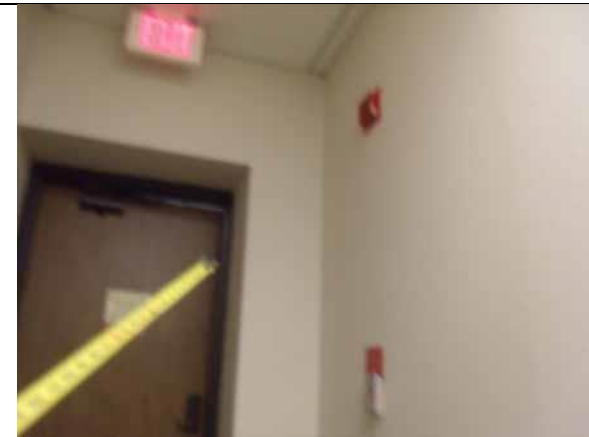
Provide proper stair exit braille signage
