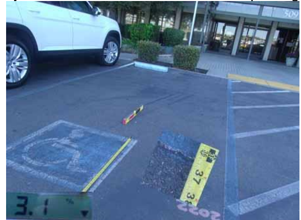
This section of slope exceeds 2.08% maximum allowed
