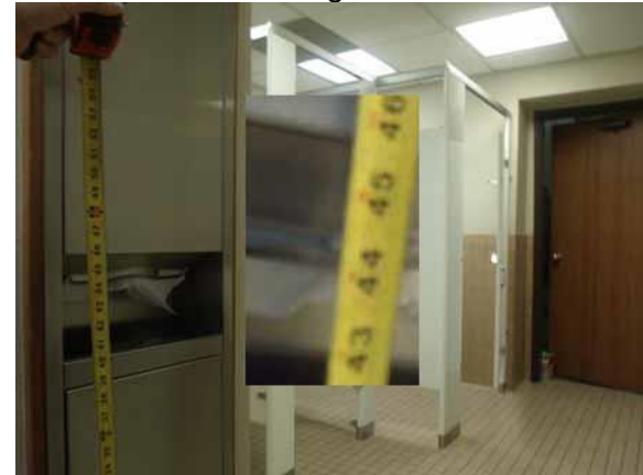
This dispenser exceeds 40" high to operable parts
