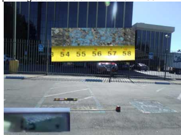
This accessible parking access aisle width is not 60" wide to center of lines
