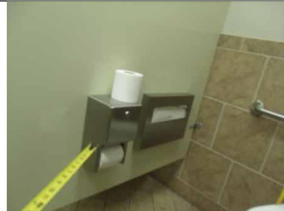
Properly locate the toilet paper
