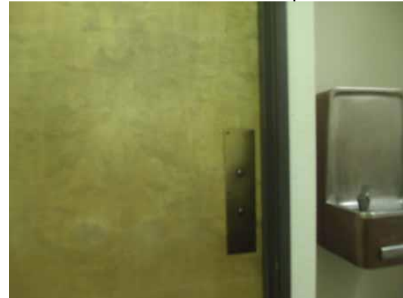
Provide proper barrier for the drinking fountain
