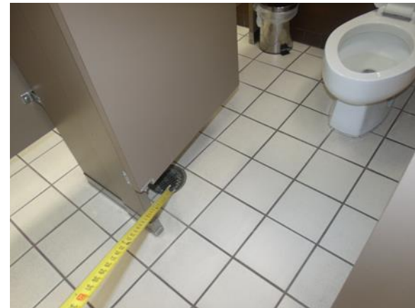
Repair the floor slope where it exceeds 2.08% maximum slope
