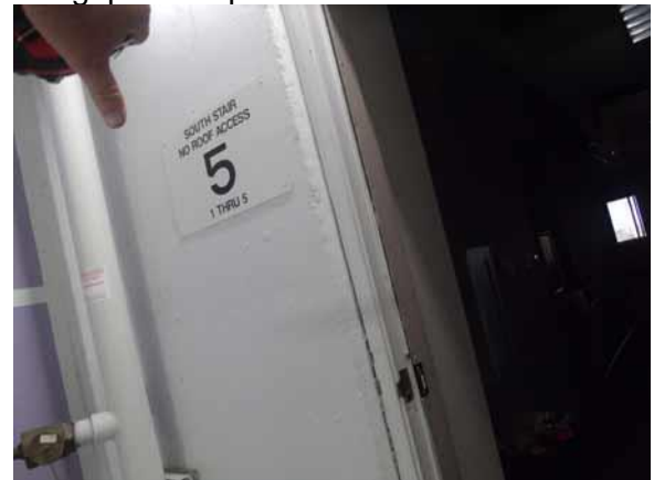
Floor identification sign is not compliant
