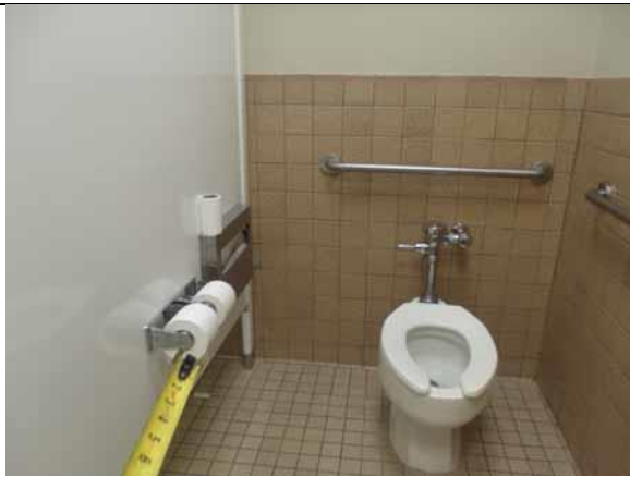
Properly locate the toilet paper
