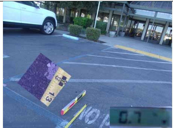
This section of slope and letter height are compliant
