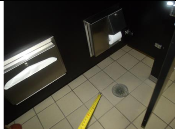
Repair the floor slope where it exceeds 2.08%
