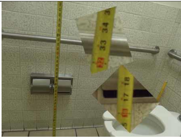
Toilet paper is not 19" minimum high
