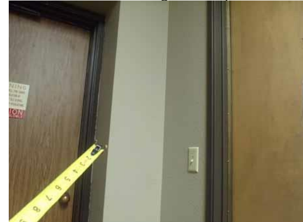
Provide proper exit stair braille signs
