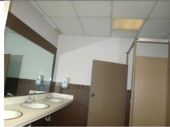
Overall lav area
