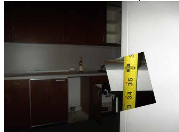
This counter height is compliant with ADA standards
