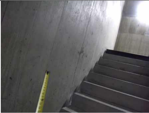
Provide proper handrails and handrail extensions
