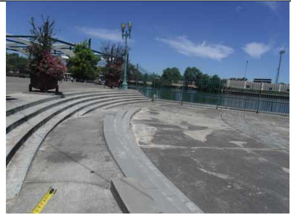
This ramp does not have handrails
