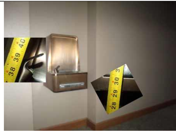
The drinking fountain spout exceeds 36" high and no high type fountain
