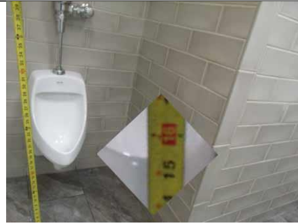
This urinal height is compliant
