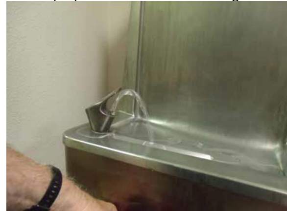
The drinking fountain water height is not compliant
