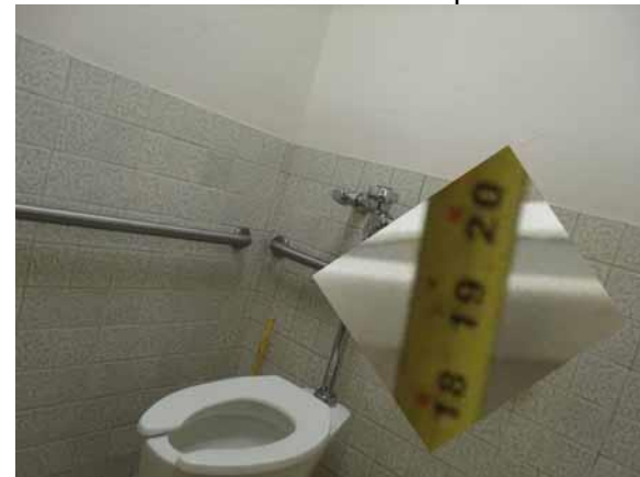
This toilet seat height exceeds 19" high
