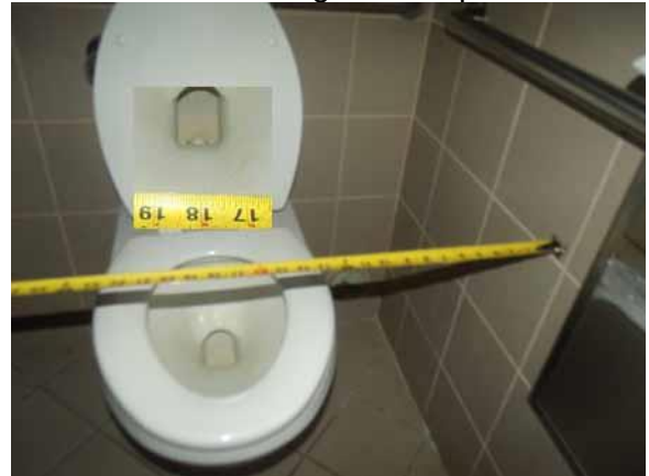
This toilet offset is compliant
