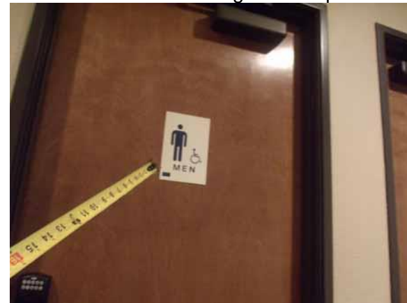
Provide proper door sign
