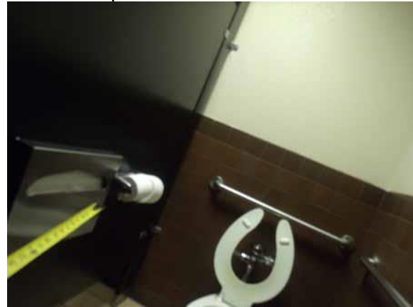
Properly locate the toilet paper
