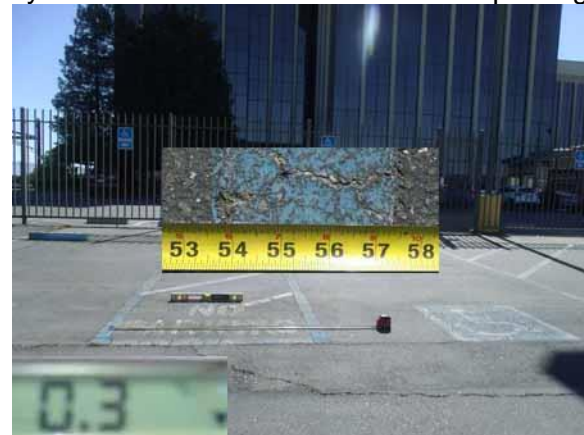
This accessible parking access aisle widths are not 60" wide to center of lines
