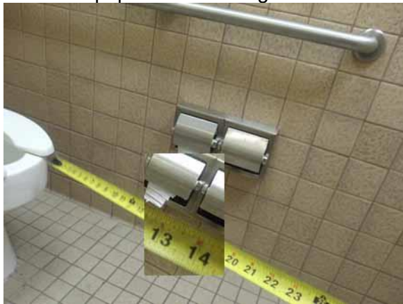
Properly locate the toilet paper
