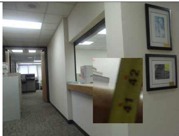
This counter height exceeds allowable
