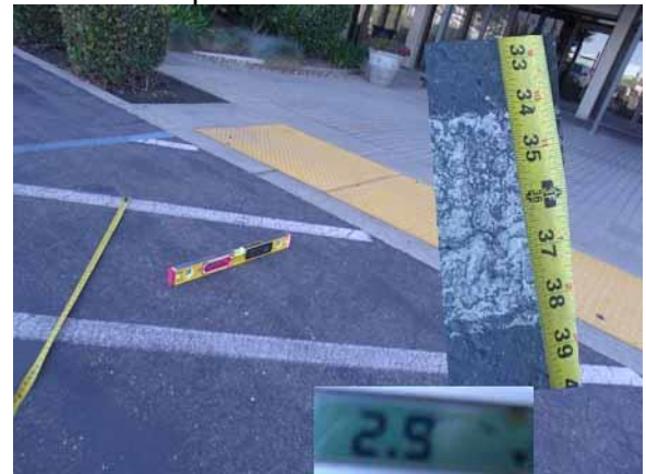
This section of slope exceeds 2.08% maximum allowed
