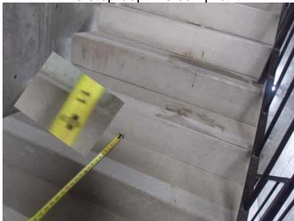
The step depth is compliant
