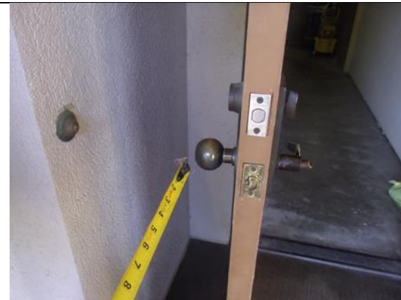
Provide proper door handle
