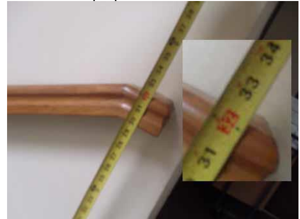
This handrail height meets applicable code
