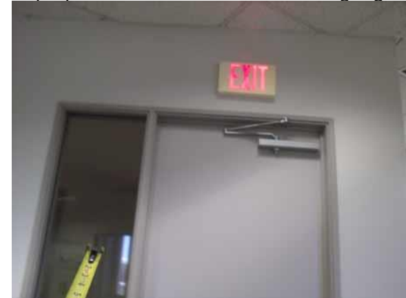
Provide proper exit braille signage Typical
