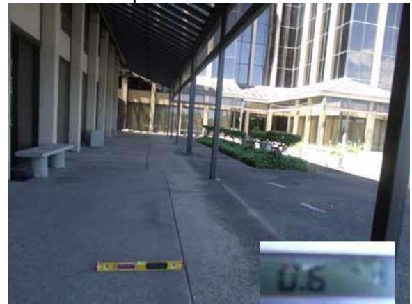
This section of slope and width are compliant
