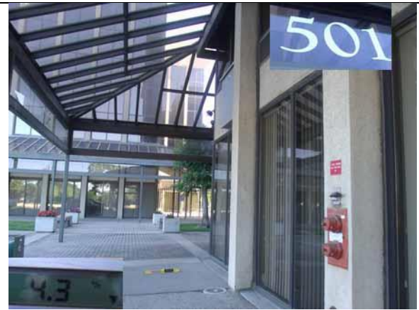
This section of cross slope exceeds 2.08%
