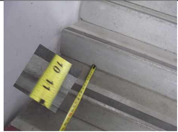
The step depth is compliant
