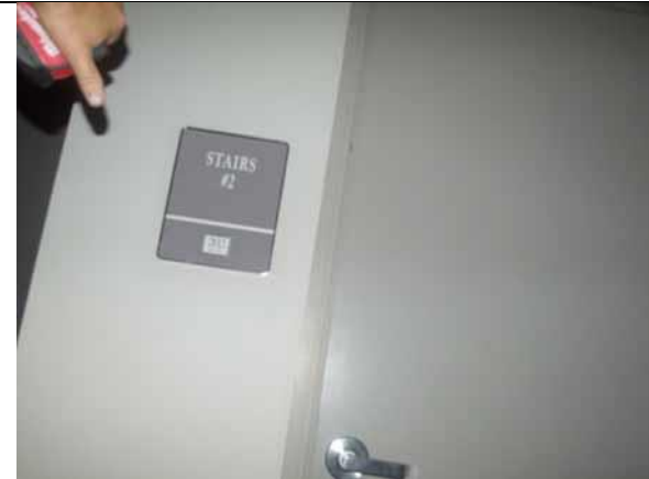
Provide proper stair exit braille signage Typical
