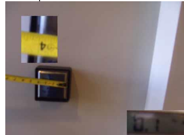
This push pad is compliant
