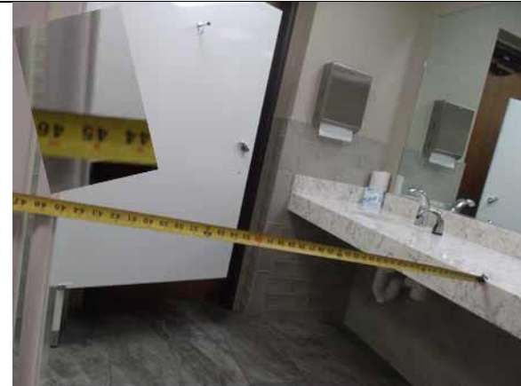
This clear area in front of the door shall be 48" minimum
