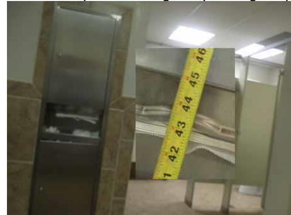
This dispenser height exceeds 40" to operable parts
