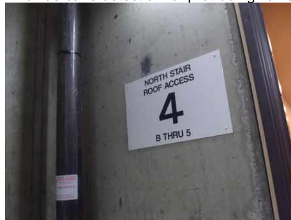
Provide proper floor identification signage
