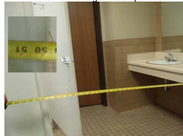
This width is compliant
