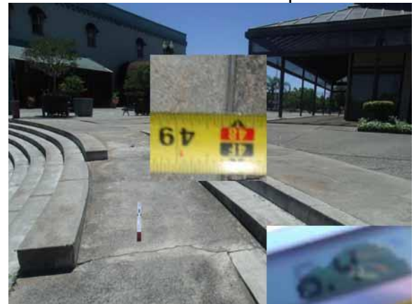
This ramp does not have handrails
