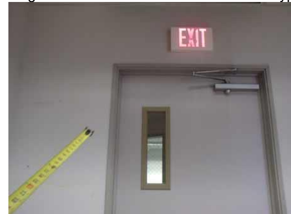
Provide proper stair exit braille signage Typical
