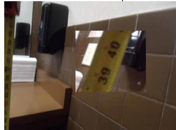
This soap dispenser location is compliant
