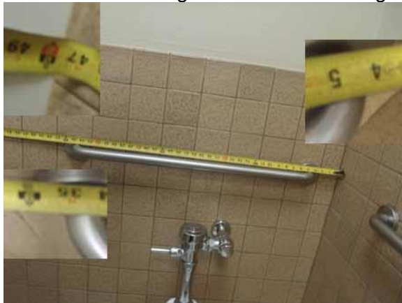
This stall width and grab bar location are not compliant
