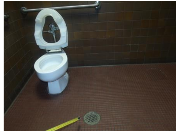
Repair the floor slope where it exceeds 2.08% slope
