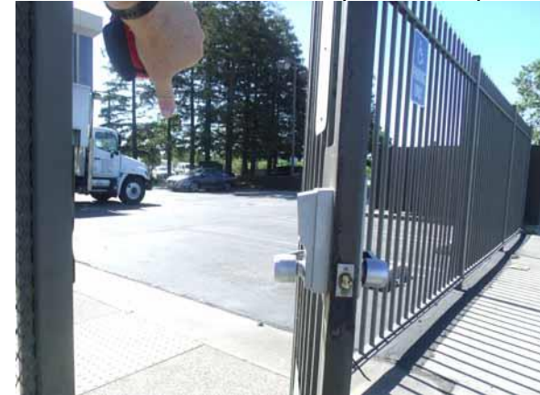
This door closing speed exceeds allowable
