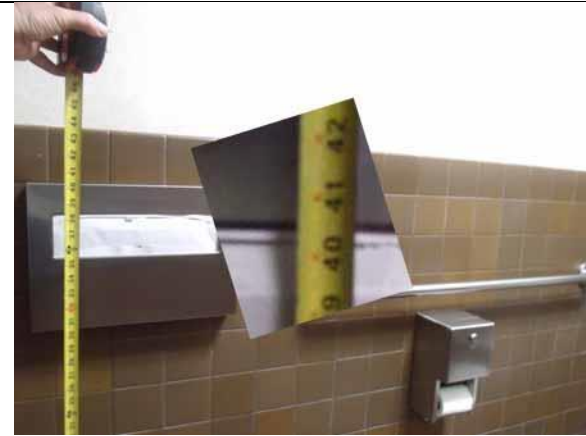
This toilet seat cover dispenser location is compliant
