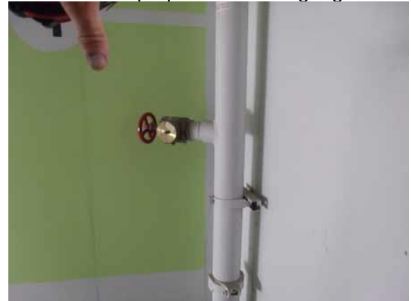
Provide cane detection under the fire riser valve
