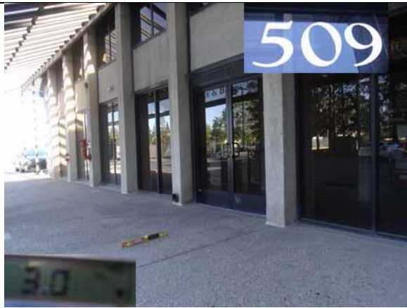
This section of cross slope exceeds 2.08%
