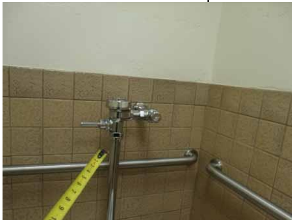
This plumbing obstructs the grab bar
