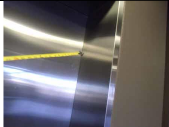
There is no 2" star for ground floor on the elevator door jambs
