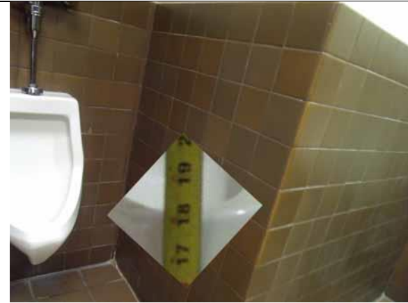
This urinal exceeds 17" high to the rim
