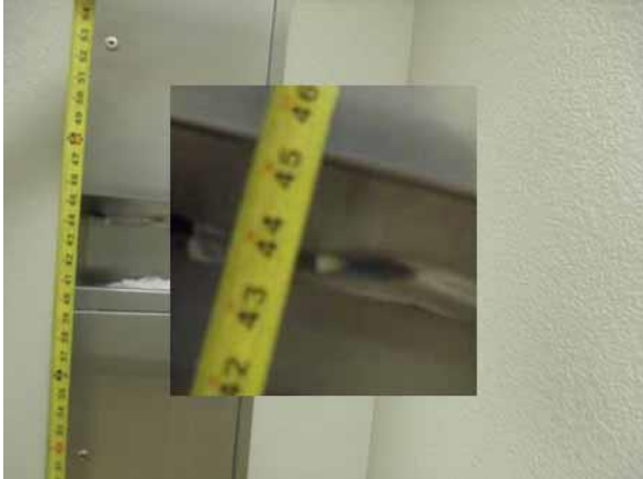
This dispenser exceeds 40" high to operable parts
