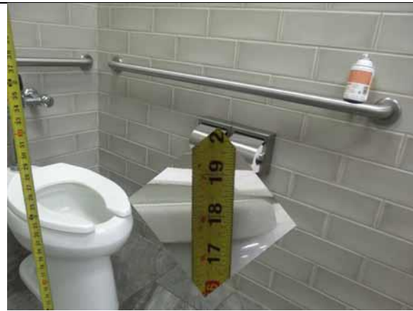
This toilet seat height is not compliant
