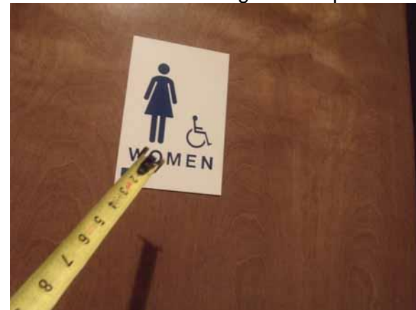
Provide proper door sign
