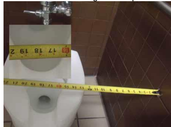
This toilet offset is compliant
