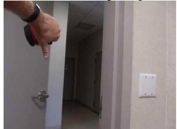
This door operation forces is not compliant
