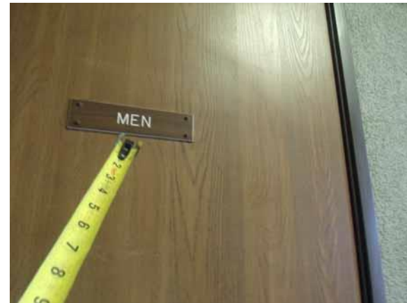
Provide proper door sign
