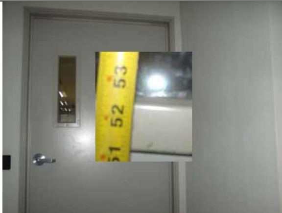
Viewing windows exceed 43" above the floor typical
