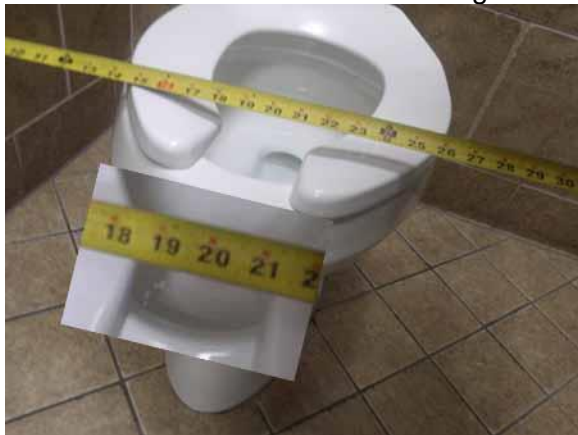
This toilet offset exceeds 18" to center from the wall
