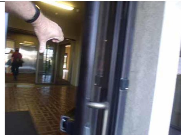
This door operation forces exceeds allowable
