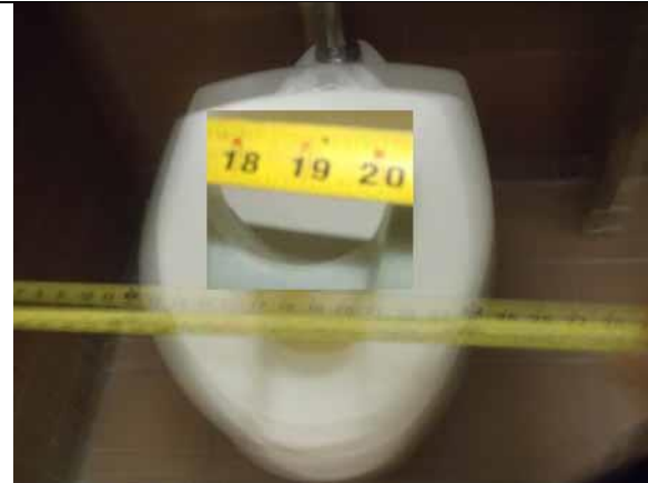
This toilet offset exceeds 17"-18" to center from wall
