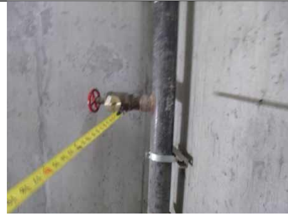
Provide cane detection under protruding connection
