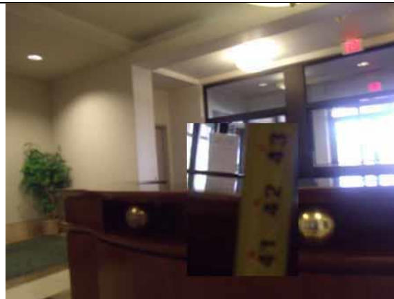
This counter exceeds 34" high
