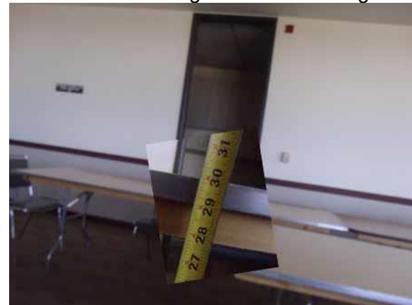
This table height is compliant
