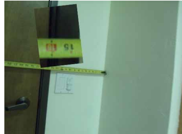
This side clearance is not 18" minimum
