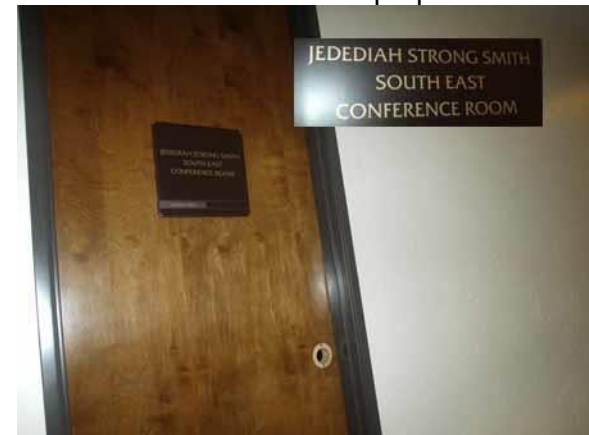
Provide proper Braille signage
