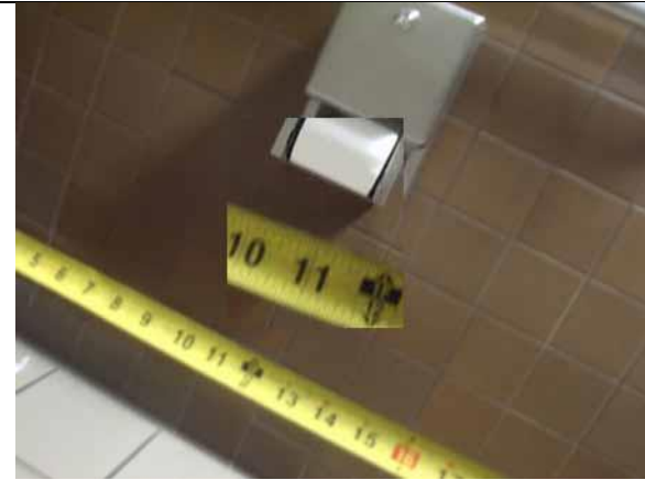
Properly locate the toilet paper
