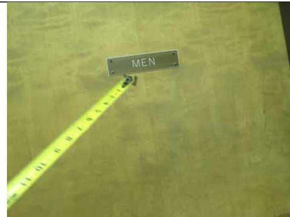
Provide proper door signage
