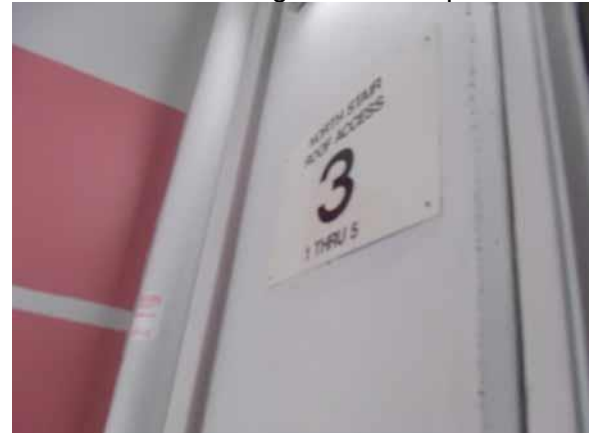
Provide proper stair braille signage
