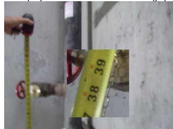
Provide cane detection for protruding valve
