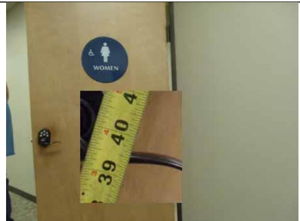
This door handle height is compliant
