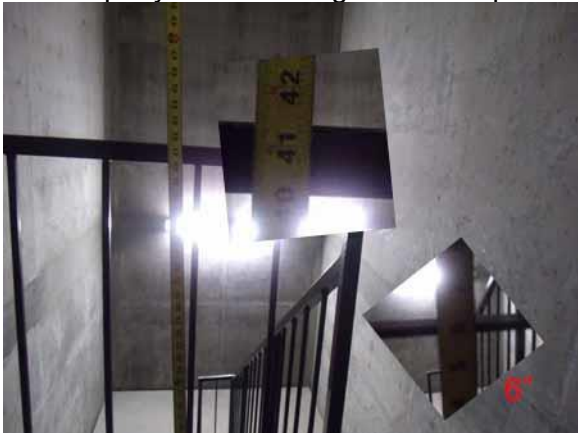
This guard rail height is not 42" high
