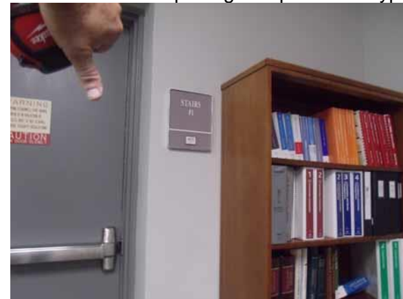
This stair exit sign is not compliant
