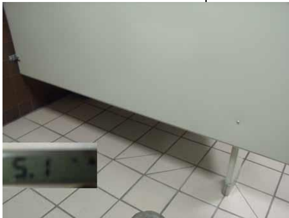
This floor slope exceeds 2.08% maximum allowed
