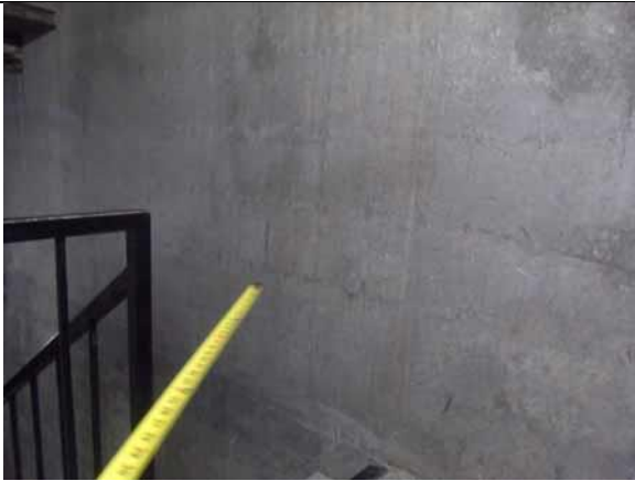
Provide proper handrails and handrail extensions
