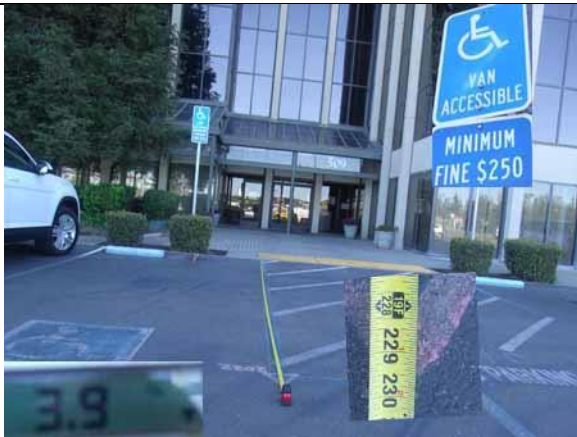
This section of slope exceeds 2.08% maximum allowed
