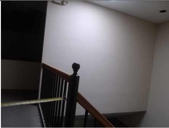
Provide proper handrail extensions
