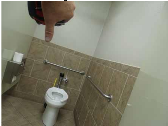
This stall is not compliant
